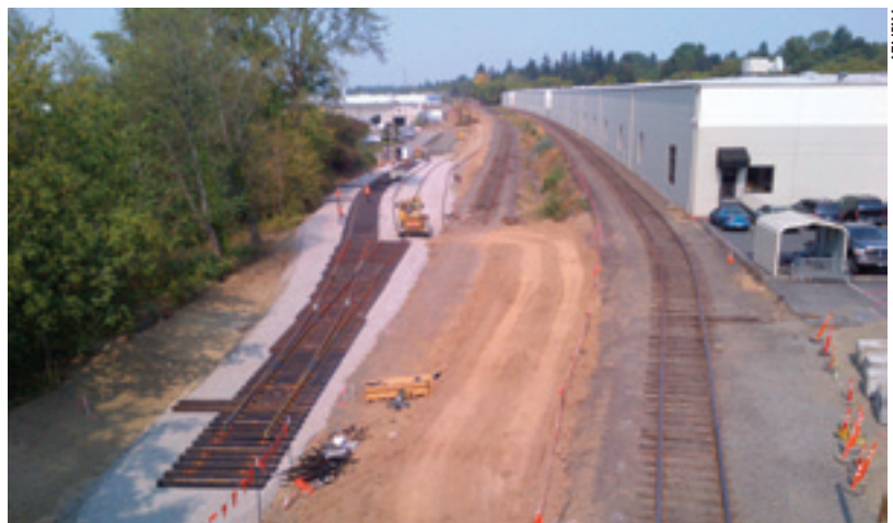
TriMet is working with Union Pacific Railroad to relocate the Class I's Tillamook branch line, located in an industrial area of Milwaukie.
